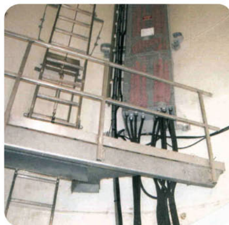
FGM风电管型母线槽系统在塔筒底端 The FGM wind-power tubular busway system is located at the bottom of the tower
